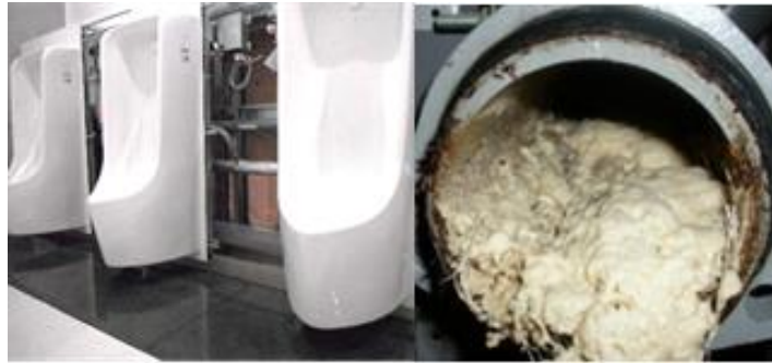
Photograph 1 – Horizontal branch drainpipe of multiple urinals and calcified urine deposited in the drainpipe
