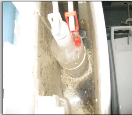
Figure 2: Visual aspect of the interior of the toilet cistern after 6 months of use [3].
