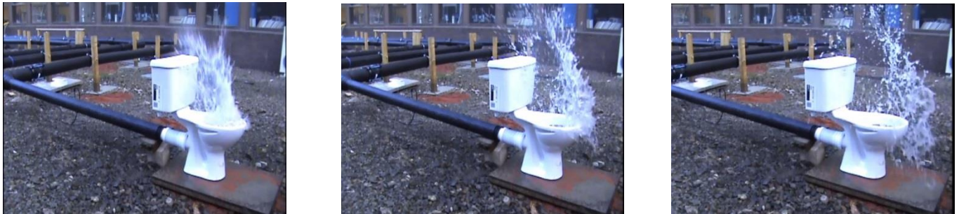
Figure 11: The effect of large pressure surge on a WC situated 3 floors from base of stack with no alleviation.
