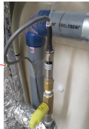
Photo 6 Water pressure measuring point
