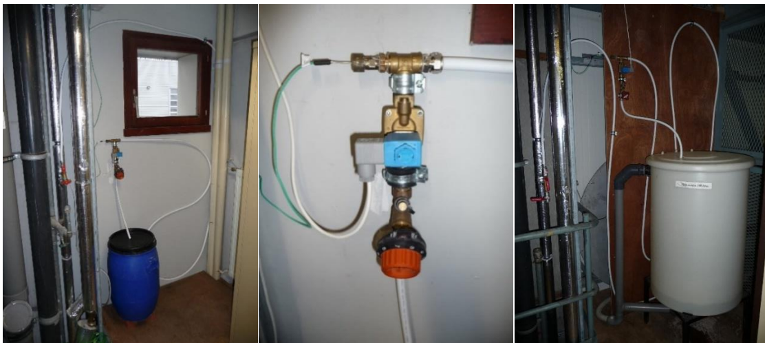
Figure 5 - views of the 'kitchen' draw-off (on the left); the 'shower' draw-off (center) and their equipments : temperature probe; electro valve and regulating valve at the reservoir connections (on the right).
